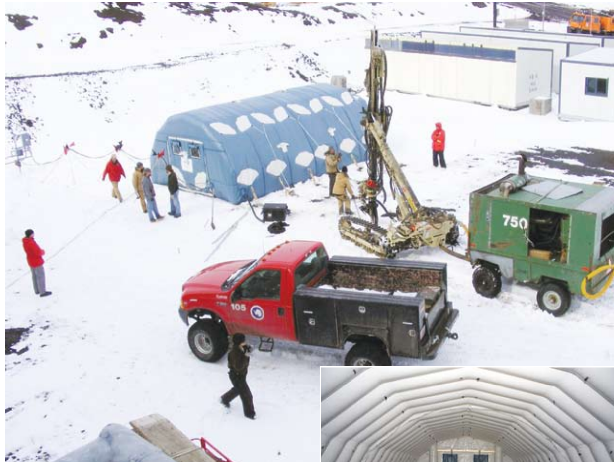
A joint project among NASA, the National Space Foundation, and ILC Dover continues at the McMurdo Complex in Antarctica. Team members drill into the tundra to install a weather station adjacent to the inflatable habitat in the upper left portion of the image.
