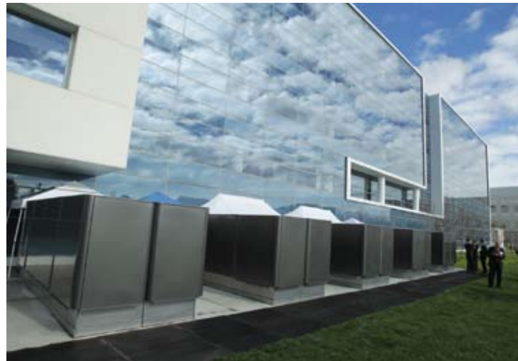
Bloom Energy Servers, seen here on eBay’s corporate campus, are now providing environmentally friendly, cost-saving energy to a number of Fortune 500 companies.
