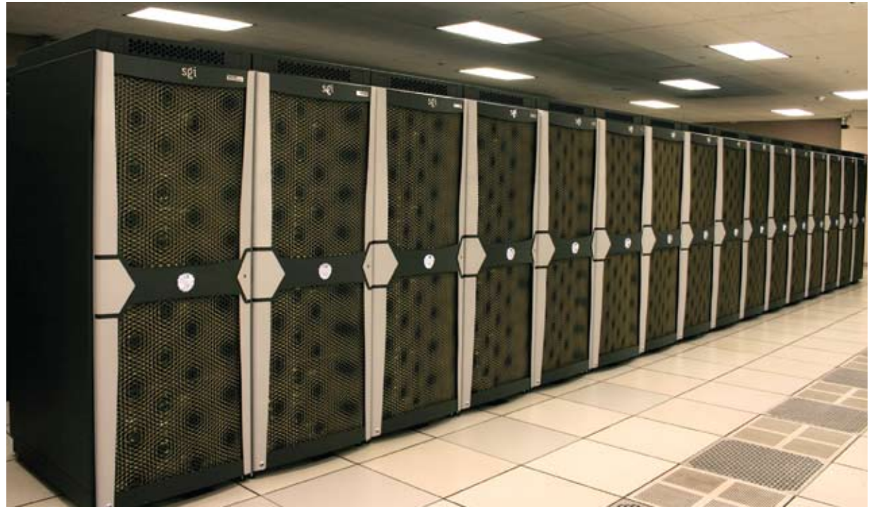
Shown here is one row of cabinets that make up the 100-cabinet Pleiades supercomputer system at Ames Research Center. In 2010, Pleiades ranked as one of the fastest systems on the Top 500 list of the world's most powerful supercomputers.
