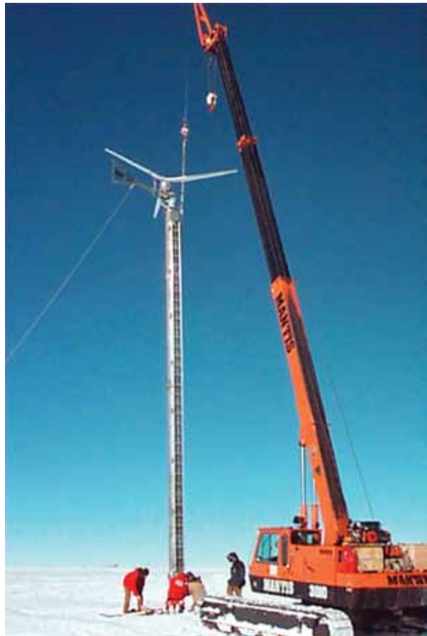
Ames Research Center provided funding for Northern Power Systems to construct a wind turbine at the South Pole, a test environment for assessing technology for use on Mars.
