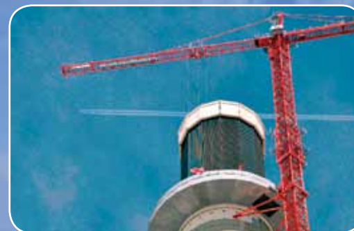
Thousands of mirrors called heliostats (top inset) are being installed in a 1,500-acre field (middle inset) to direct the Sun's energy onto a receiver (bottom inset), which was built using expertise gained from constructing the SSME. The NASA spinoff receiver will sit on top of a 550-foot tower (background image). During construction, this solar power project will generate more than 4,300 jobs.
