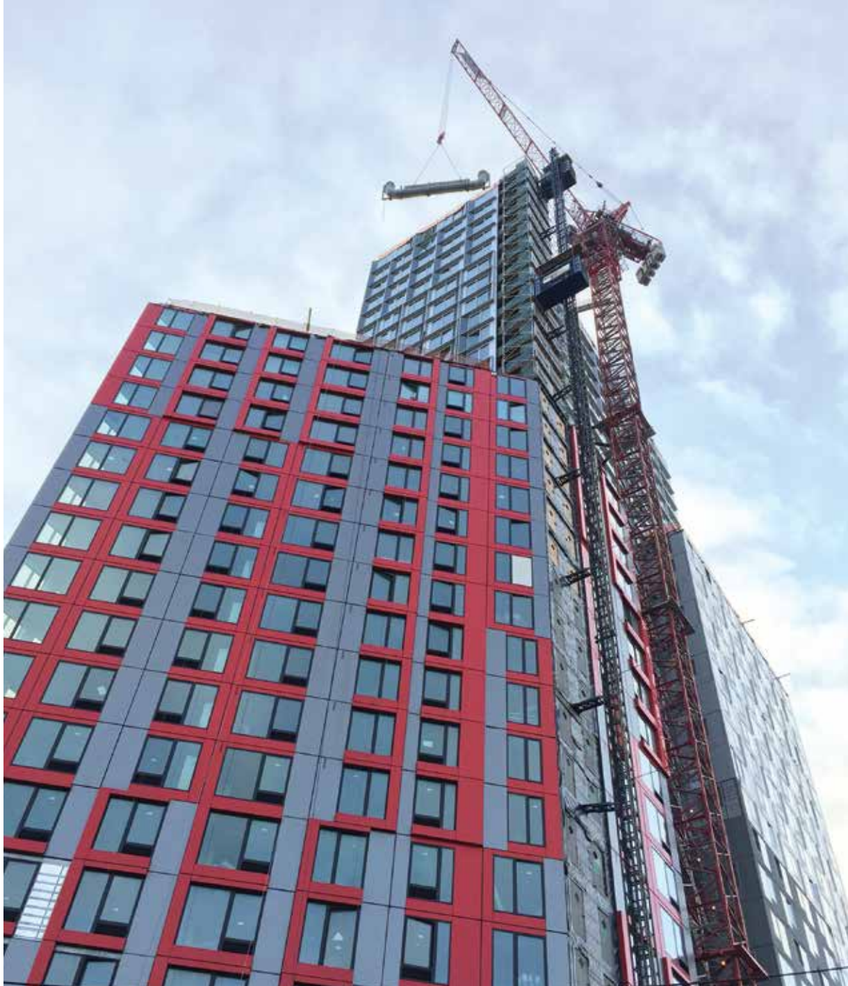
Engineering firm Thornton Tomasetti has licensed the disruptive tuned mass damper technology for commercial use in buildings and bridges. Here a crane lifts a damper to the roof of B2 BKLYN, the first project they are using the NASA-derived technology on.
