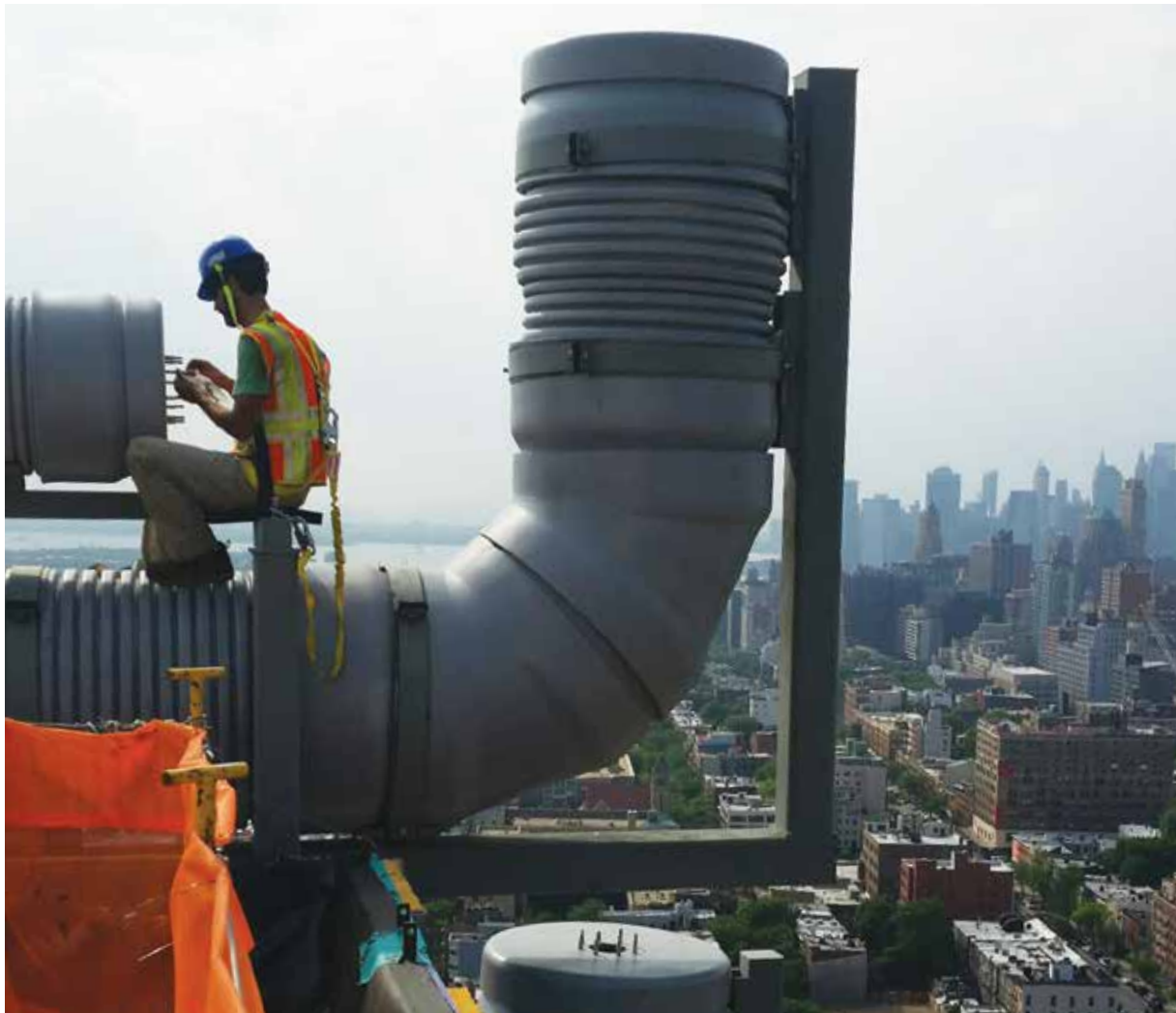
The NASA-developed devices are installed in four specially designed water-filled pipes along the roof of B2 BKLYN. The damper, which Thornton Tomasetti is marketing as Fluid Harmonic Dampers, is cheaper and more flexible than previous vibration dampening options.
