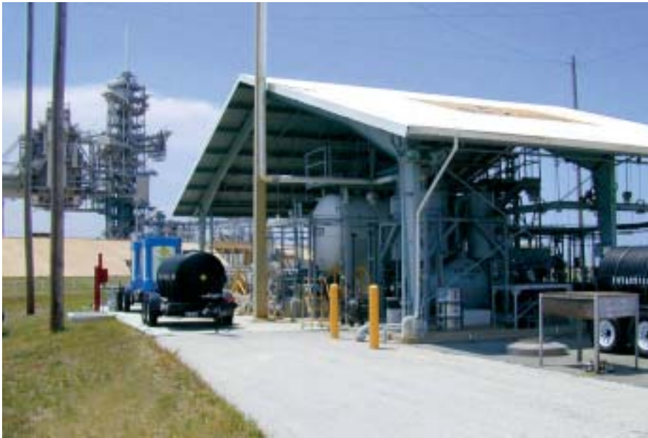
The NOx Scrubber Liquor to Fertilizer system installed at Shuttle Pad 39A at Kennedy Space Center.
