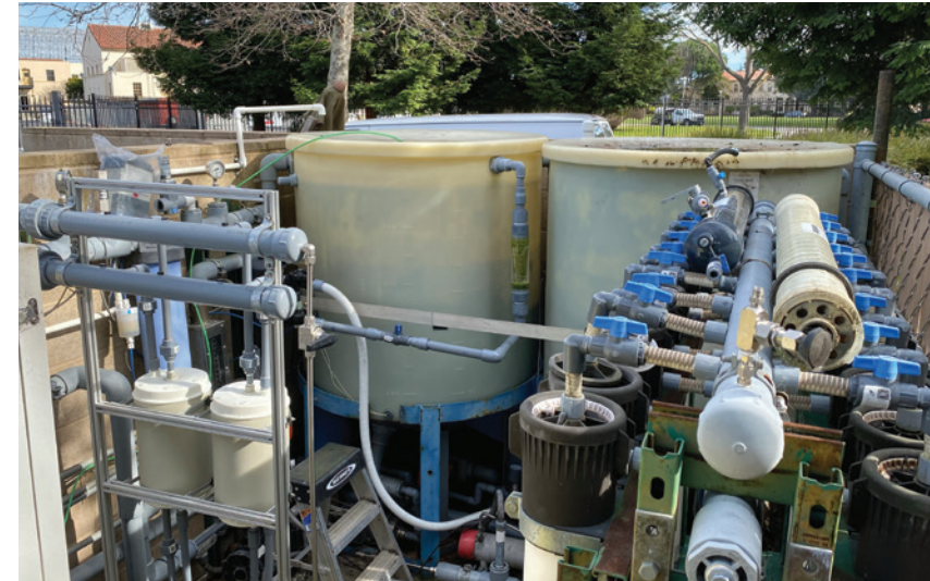
In the gray water reclamation system at Ames Research Center's Sustainability Base, the two beige Aquaporin HFFO14 forward-osmosis modules on the left have as much filtration capacity as the entire legacy system on the right. Credit: Aquaporin A/S
